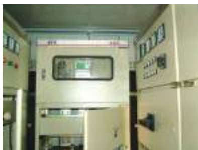
Secondary Cells Room
